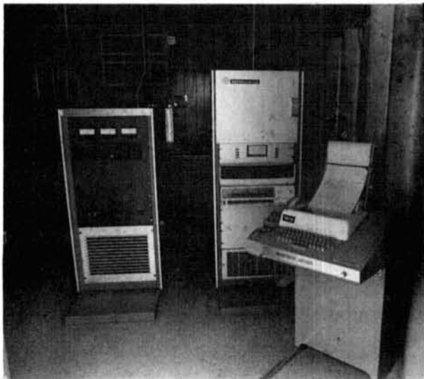
fig. 6. Interior of master station at Boise, Idaho.
